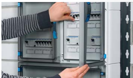
■ Hand-operated doors in areas to which unskilled persons have access for operating devices
