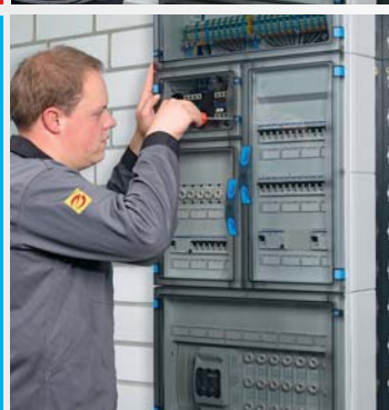
Access and operation only by electrical skilled persons
