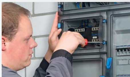
■ Tool-operated doors in areas to which only an electrical skilled person may have access
