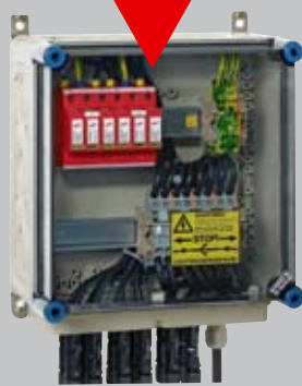
PV generator junction boxes
