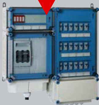
PV Solar inverter collector
