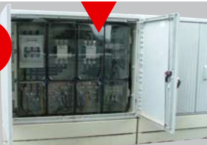
Disconnection, metering, overcurrent protection device
